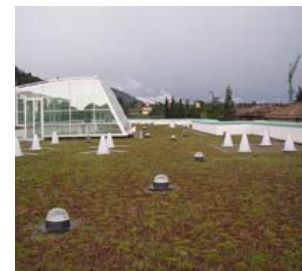
View of the terrace at the top of the hospital with sun-pipes and light ducts
