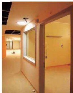
Sun-pipes installed in front of patient rooms
