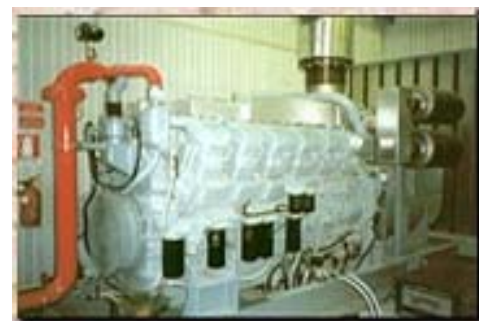
The CHP plant installed in the Meyer Hospital
